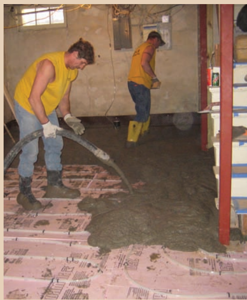
Pouring the concrete over the in-floor heat. Cozy days ahead in the Mogush basement
